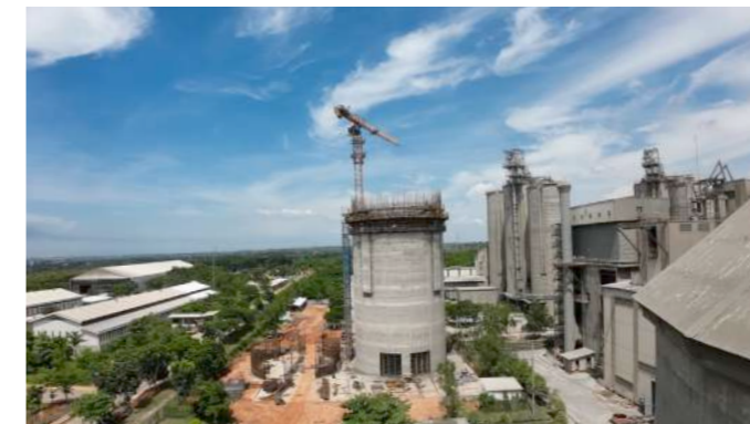
Silo Semen Tuban Indonesia | Post-tensioning strand systems
