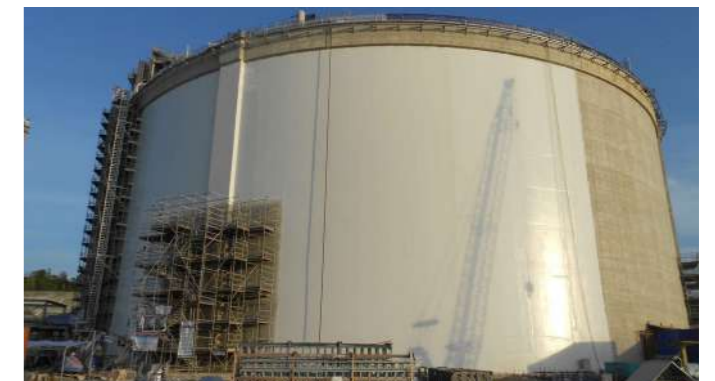
Donggi Senoro LNG Tank Indonesia | Post-tensioning strand systems
